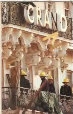
Firemen clear debris near Thatcher rooms
